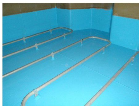
Chem-tect™ RB 300 Chemical Tank
