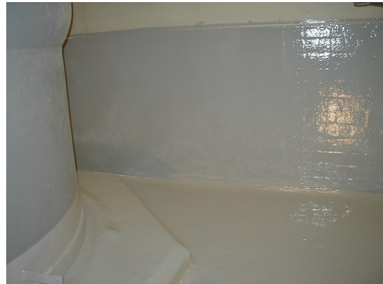
Epo-chem™ RF 500 Bund Lining
