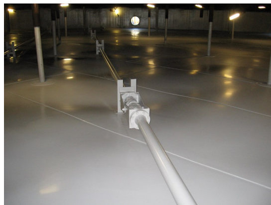
Epo-chem™ RA 500M Crude Oil Tank
